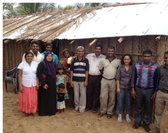
AsiaTeak Staff repaired this roof for a family with a disabled child
